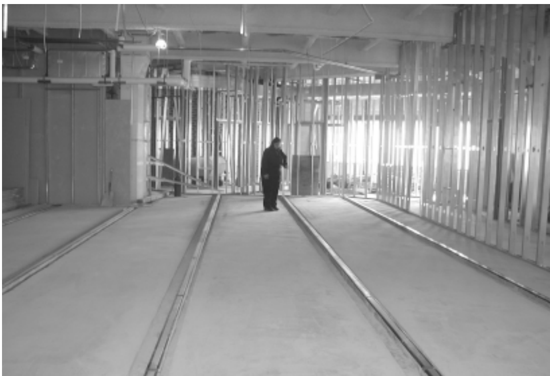
Marie Dvorzak examines newly-installed tracks for compact book shelving in the library addition of the West Wing. The shelves will contain approximately 50,000 volumes. Photo, Mary Diman.
