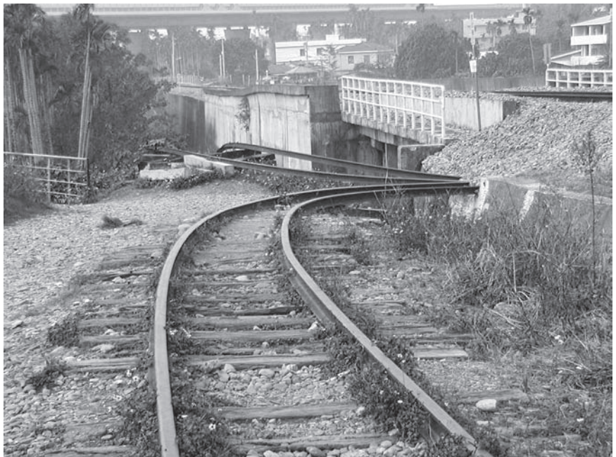
Displaced railroad tracks resulting from the 1999 magnitude 7.5 Chi-Chi earthquake. Nik took this photograph spring 2006 when he was doing fieldwork in Taiwan.
